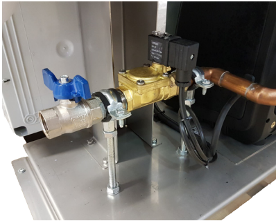
Quick fill 3/4" solenoid valve from incoming supply
