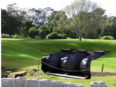
Low level interconnecting pipework
